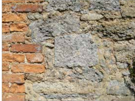
Winklestone in the west wall of Plaistow Place
